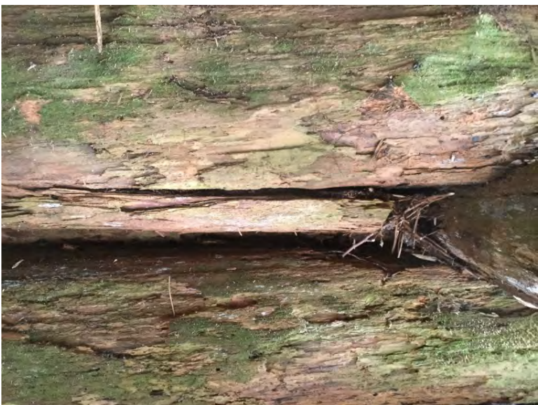
Top face log at left bank horizontal crack
