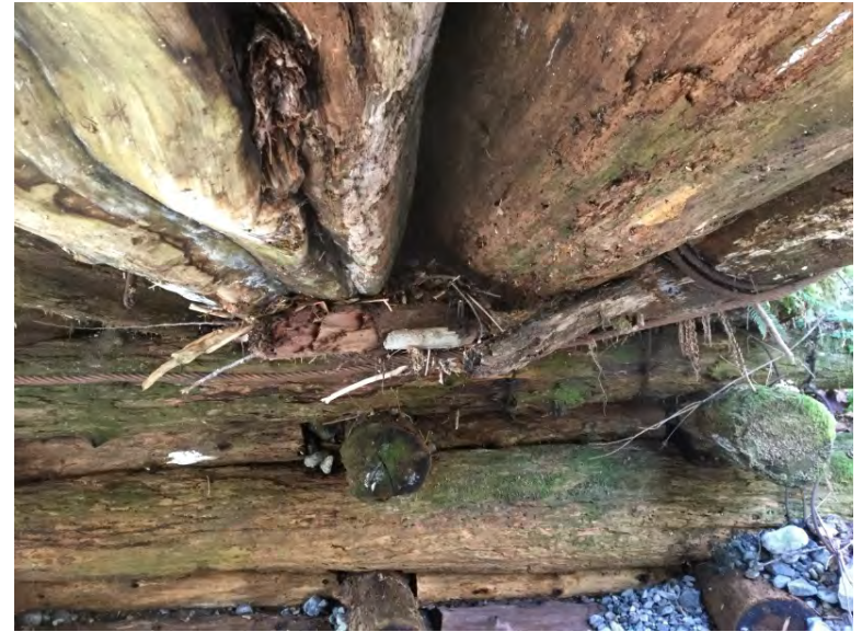
Evidence of stream flow at stringers
